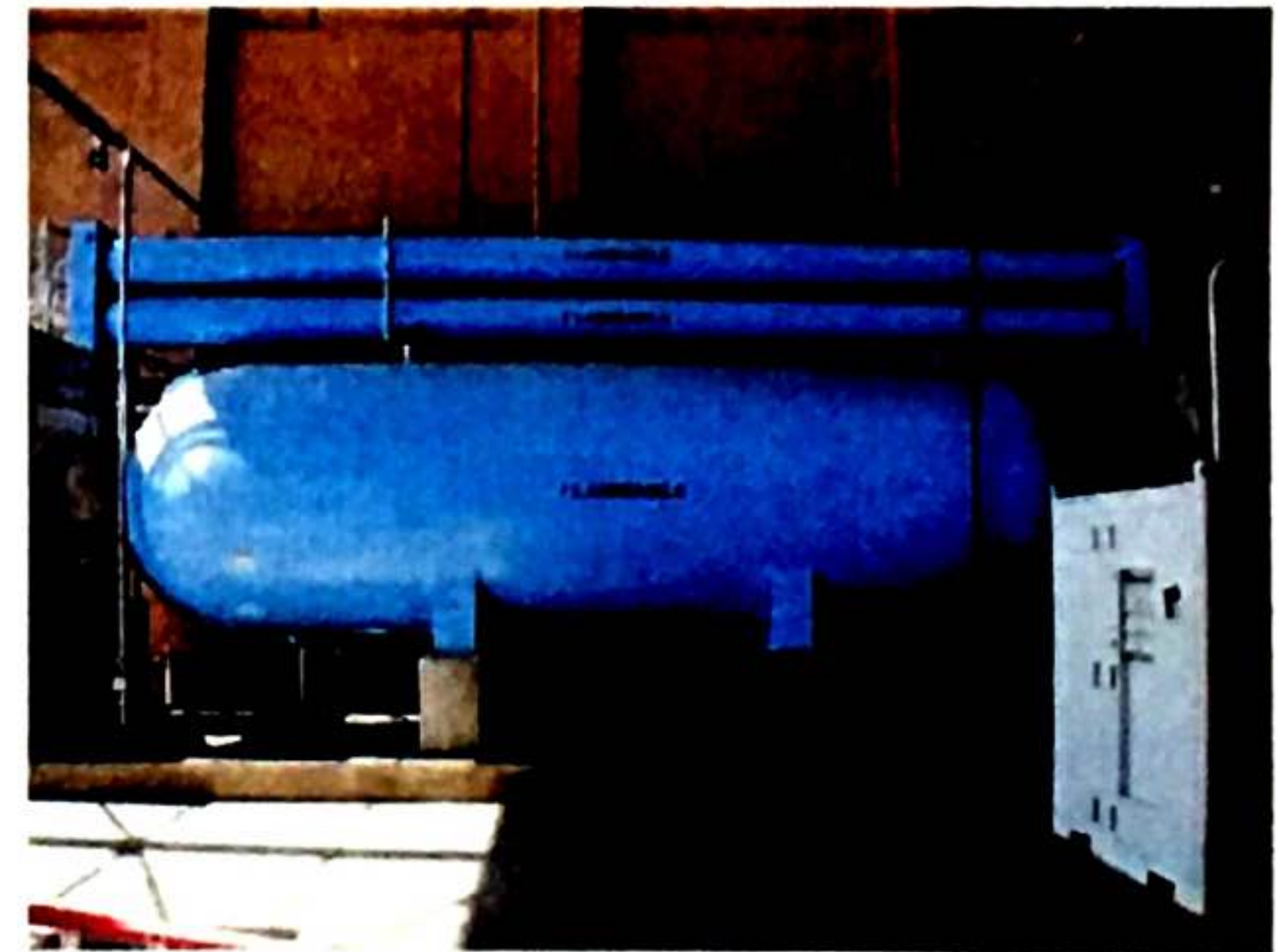
Hydrogen low-pressure storage tank, two high-pressure storage tanks, and PEM electrolyzer on right.
